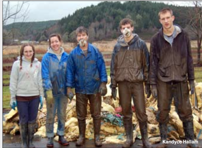
More than 50 Auburn Adventist Academy students and teachers help rip out water-soaked insulation.
