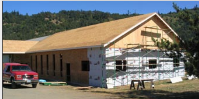
With hard work Maranatha volunteers and Winston Church members complete their sanctuary.
