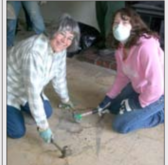
Verna Ames and Sarah Mills, Friends Helping Friends volunteers, pull out nails and staples after carpeting was removed in this home.
