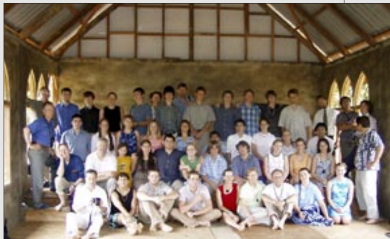
In spite of all the things that had to be done by hand, the UCA Borneo group completed this beautiful brick church in only five days.
