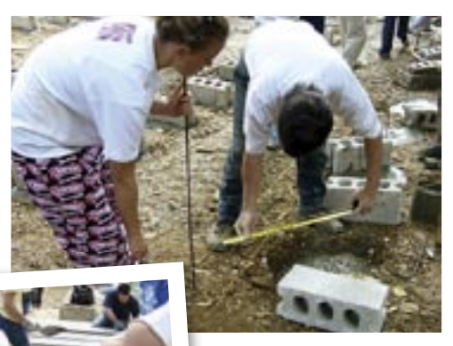
Tricia Kimbrough, AAA senior, and Keith Hallam, AAA principal, work together building at the youth camp amphitheater project in Puerto Rico.
