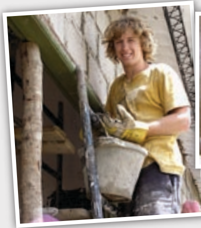
Paul Curtis works hard to patch up the spaces between the bricks and the roof.
